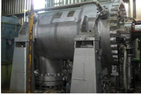
Vibration and Performance Monitoring on compressor and turbine
