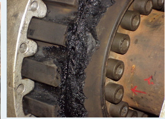
Melted rubber coupling
