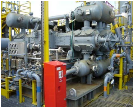
Figure 4: Example of Reciprocating Compressor on FPSO. Dynamic analysis of compressor forces on FPSO structure requires coordination between Machinery Consultant, Packager, and Engineering Consultant.
