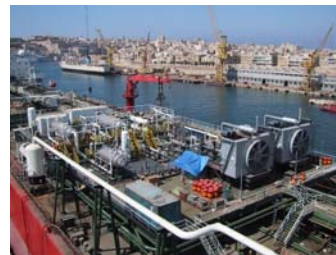
Figure 7: FPSO Design for Two 1000HP (746kW) Compressor Units on a Common Topside Structure
