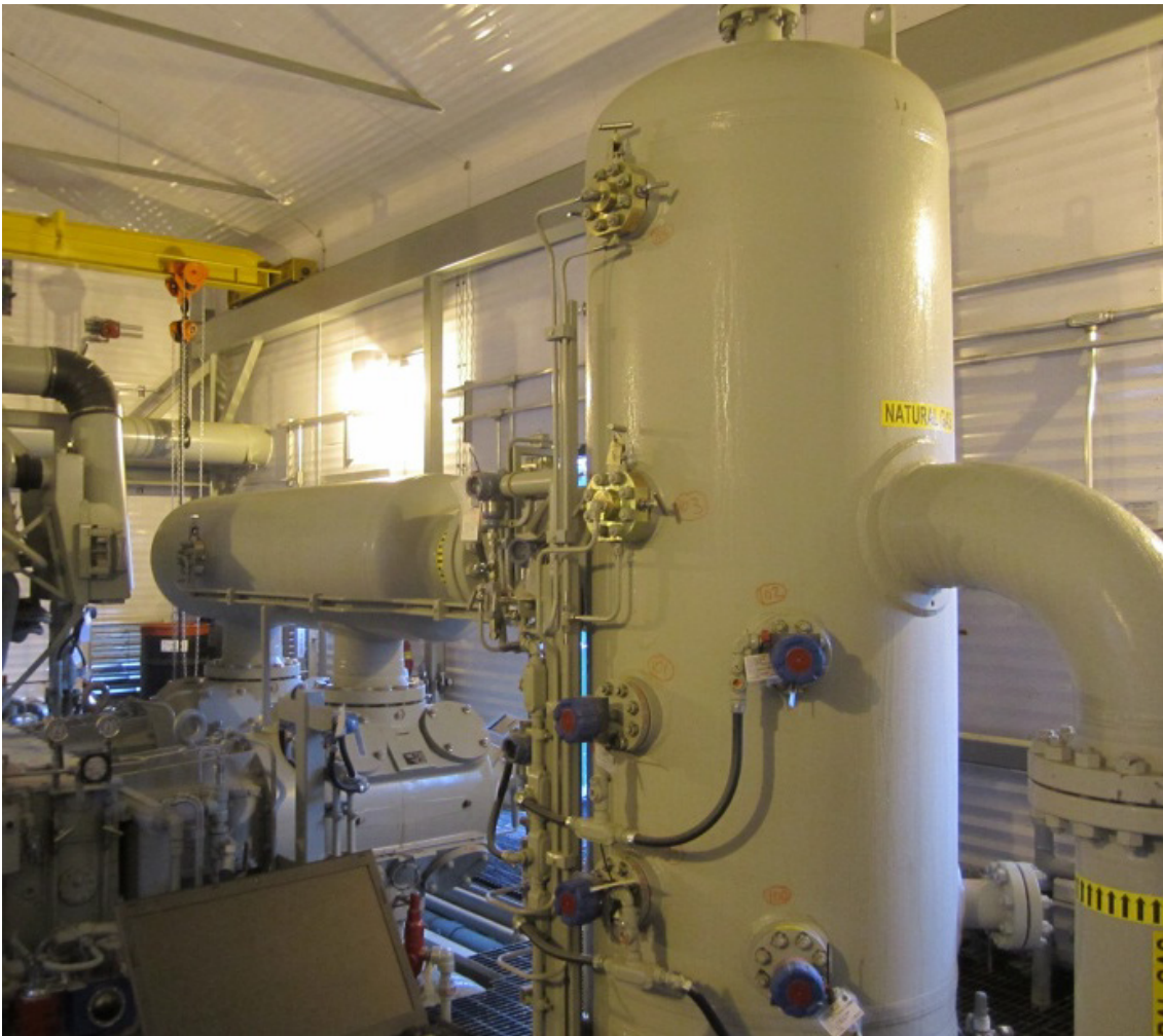
Figure 15: Robust Small-Bore Attachment Design at Sundance is the Result of Continuous Improvement and Effective End-User Specification.
