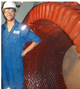
Turbine end of generator stator
